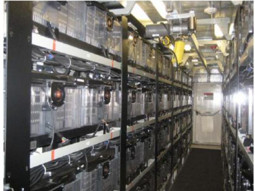
Caption: Interior view of the Altairnano battery management system
