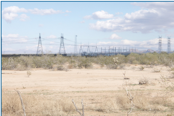
Tortolita Substation in the southern portion of the study area.
