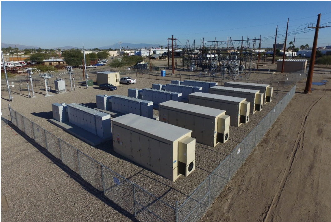
Picture 4 – 10 MW Battery Energy Storage System at DeMoss Petrie
